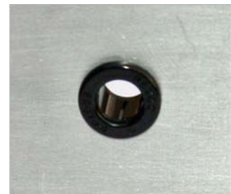
Snap Bushing Installed
